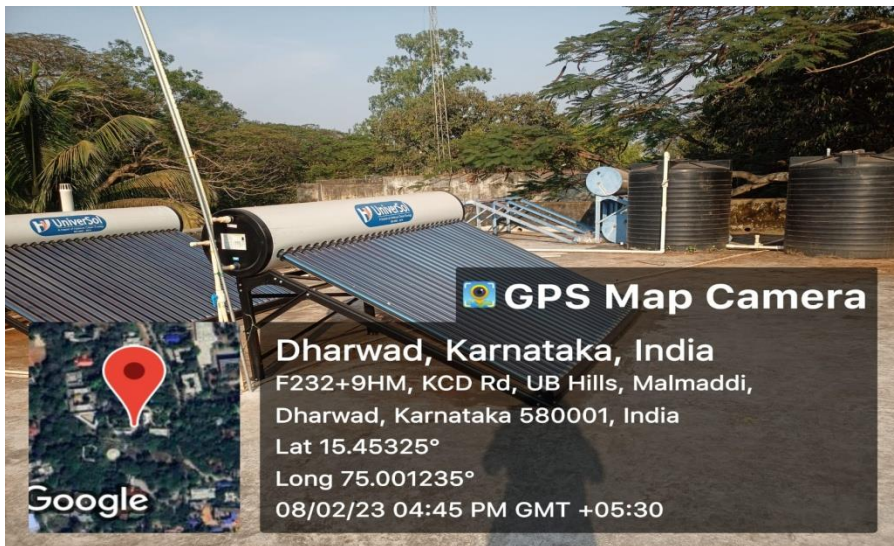
Solar heater installed in the Kaveri hostel
